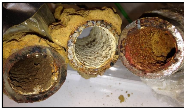
Figure (1-1): Corrosion water pipes.
